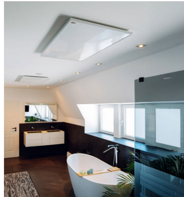
Ceiling heating in the bathroom.
